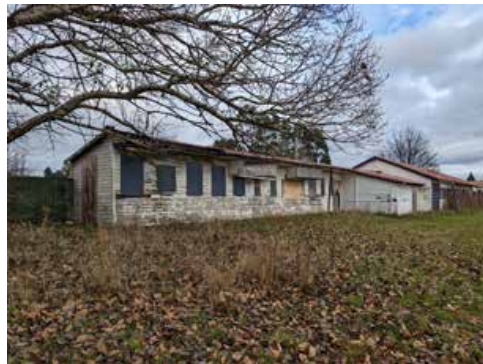
Given the state of dilapidation and the inherently low-quality building stock, much of the heritage precinct needs to be demolished.
