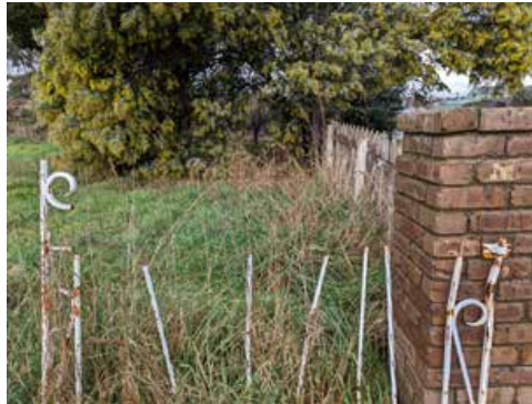
The entry gates are rated highly in the H.I.A document. However, due to vandalism and partial removal, this should be updated.
