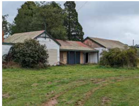
It was hoped to keep the facade of this particular building but due to the state of the dilapidation it will have to be demolished.
